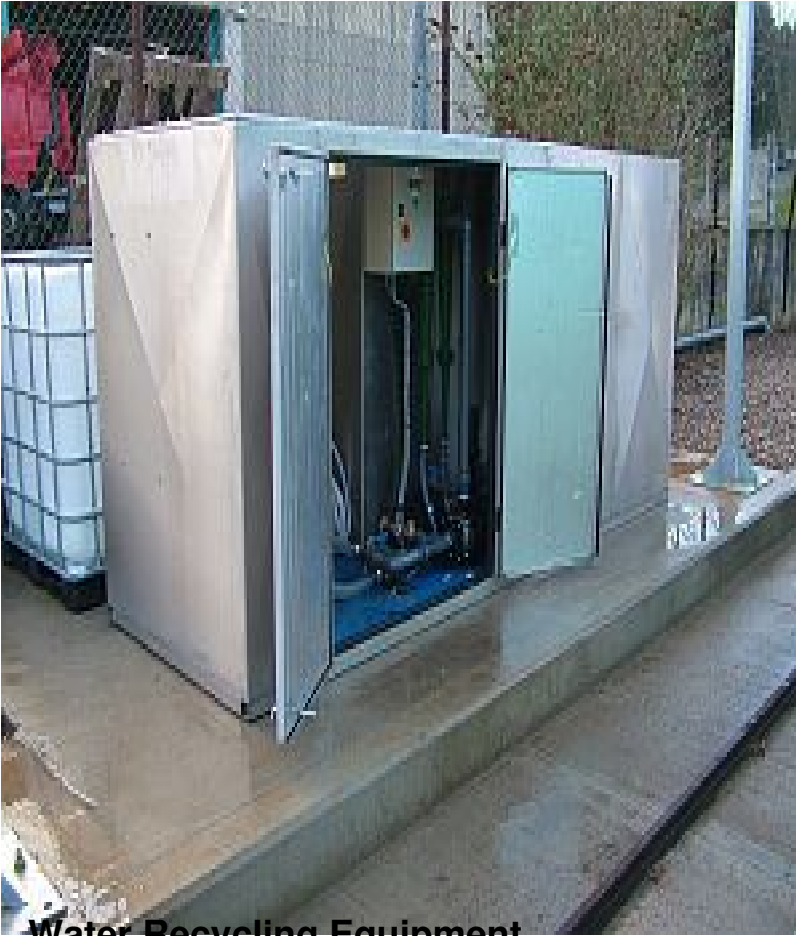
Water Recycling Equipment
